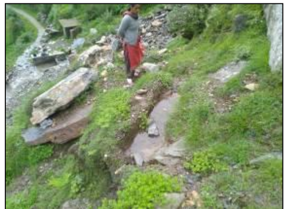
Trenches in recharge area of Kulha Malun spring, Trishun village under Rural Department
