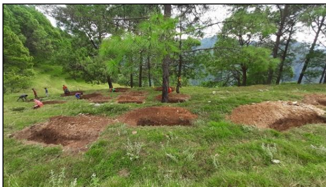
Implementation work in the recharge area of spring Successfully completed engineering and vegetative measures for 20 critical springs in Bareth (5), Malan (5), Moldhar (3), Kotigad (3), and Ghurdauri (4) watersheds, involving the excavation of 3,454 trenches in spring recharge areas.
